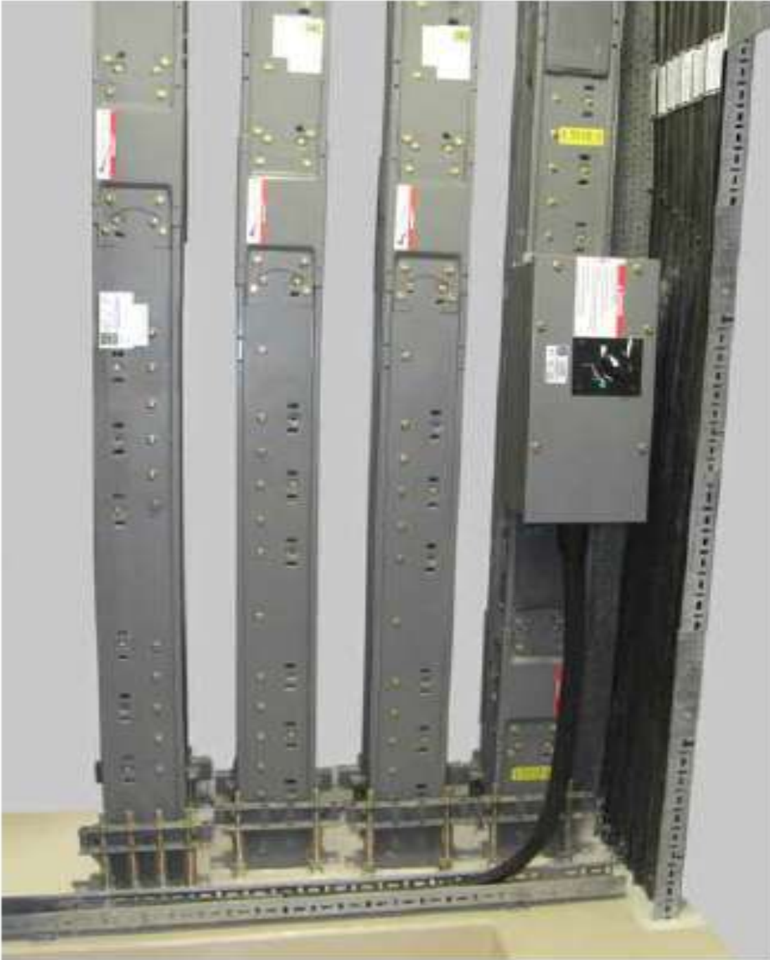
Typical busbar riser system including plug-in circuit breaker
